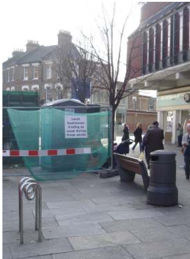
High Road - pavement obstructions
